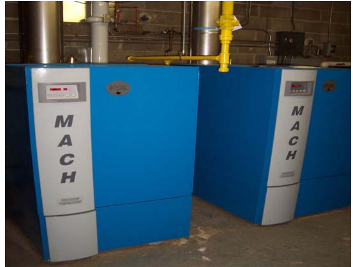
Lakewood Combined Heat and Power
