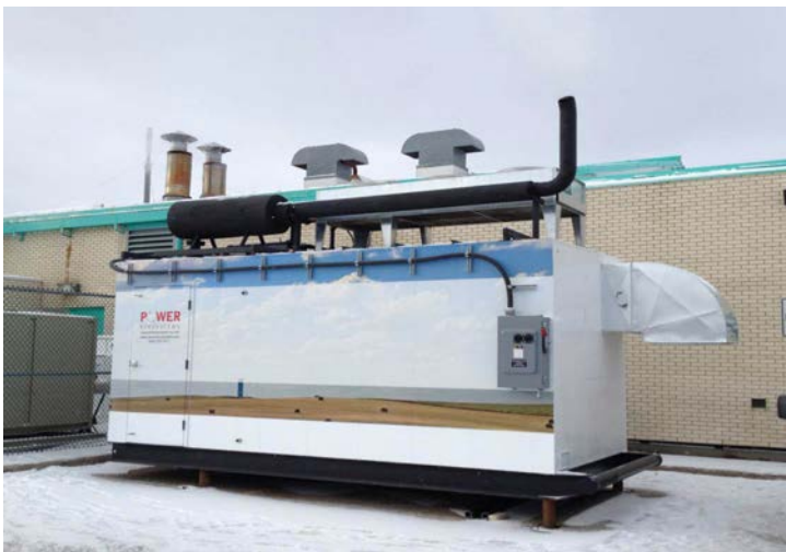
Lakewood Combined Heat and Power
