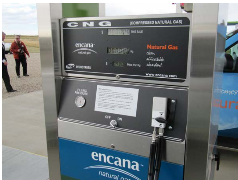
Compressed Natural Gas station
